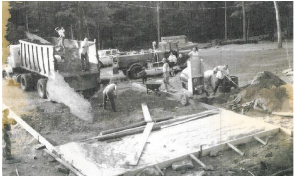
Foundation being laid for Walker Lake Volunteer Firehouse (courtesy of Deluccia family photos)
